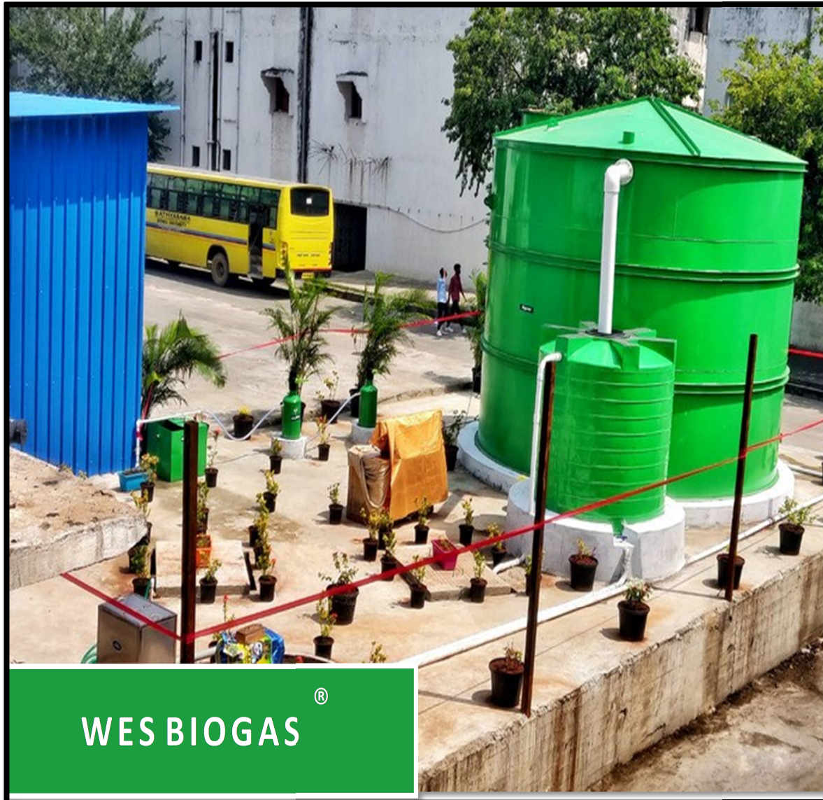
Figure 67: 1Ton/day Biogas plant Installed and Commissioned at Sathyabama Institute of Science and Technology, Chennai
