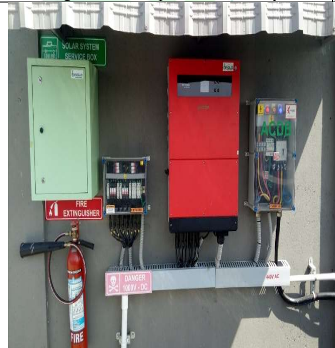
Figure 25: Solar system with Service box
