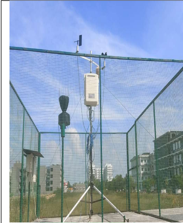
Figure 27: Solar-wind hybrid system
