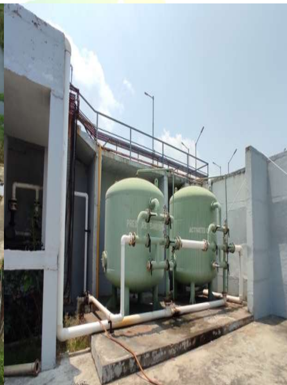
Figure 38: Water treatment unit
