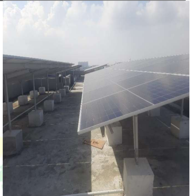
Figure 21: Rooftop Solar Panel
