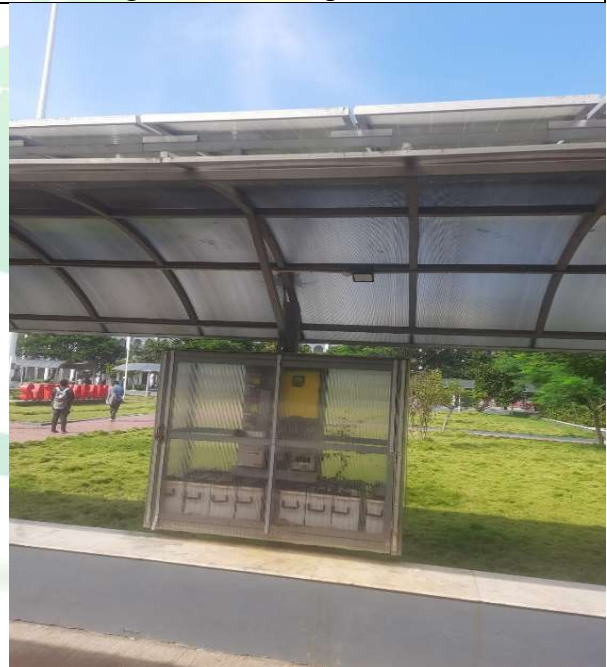
Figure 22: Solar Inverter with controller
