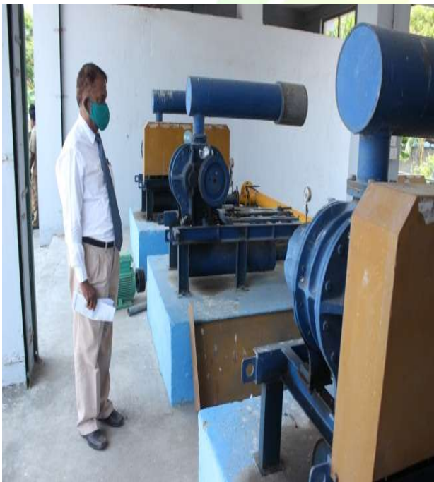
Figure 41 :Lead auditor inspecting the blowers
