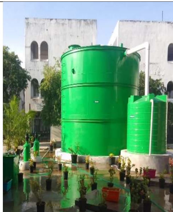
Figure 68: Biogas Digester and Slurry collection Tank
