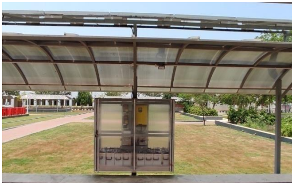
Solar panels with controller
