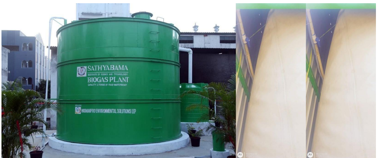
Biogas Plant with 12ft biogas collected in the balloon adjacently diverted for cooking
