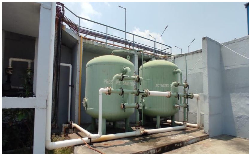
STP-Sand Filtration, Carbon Filtration
